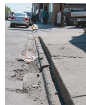
6. Deteriorating, Double-Stepped Curb and Gutter
